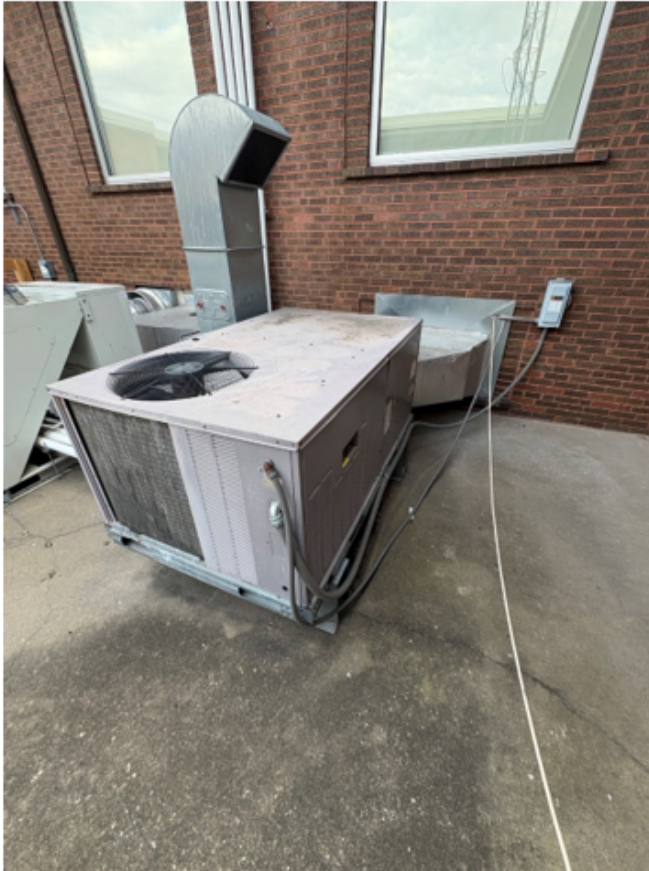
RTU #3. Cooling only unit installed in 2005. Severely undersized for area it serves (dietary & Server room where increased heat loads diminish its effectiveness and efficiency.
