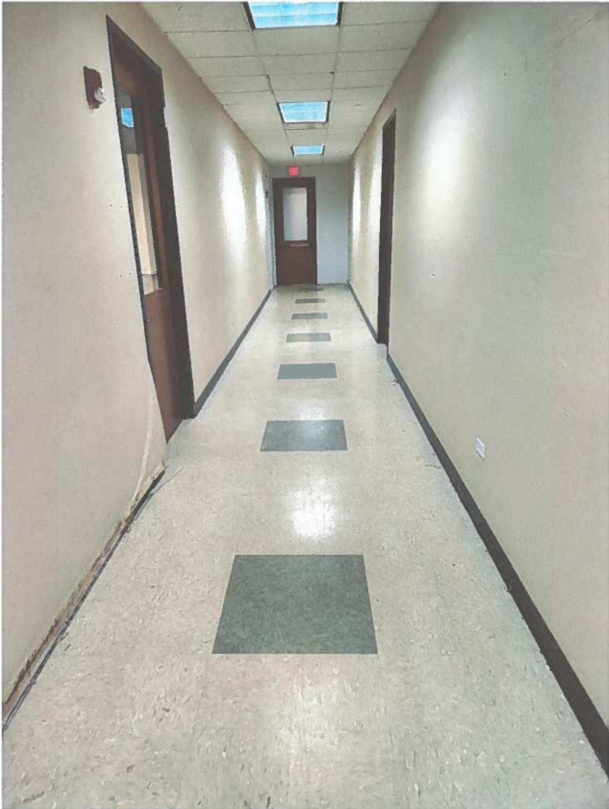
Hallway to Non-Clinical Space Acquired to Make Room for Proposed Cath Lab.
