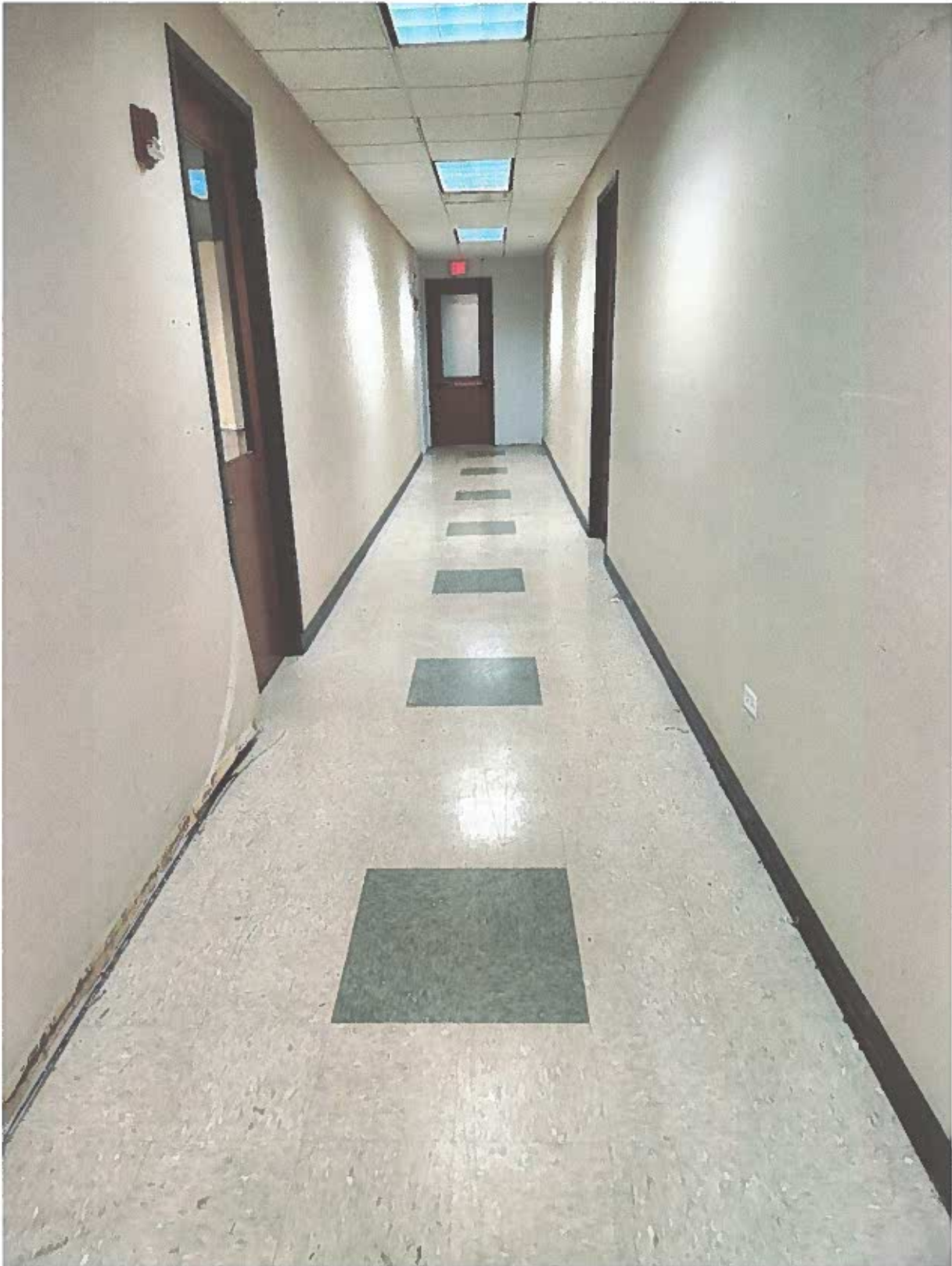
Interior: Existing Non-Clinical Space Being Converted Into Cath Lab – Hallway to Suite 110
