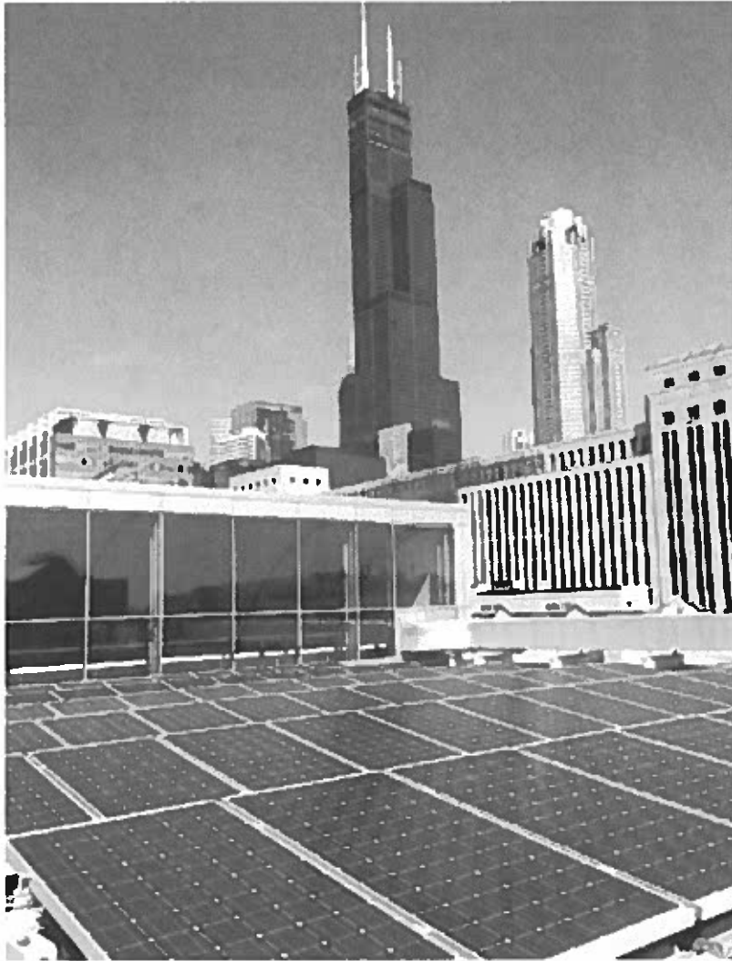
Domestic Violence Courthouse – Photovoltaic/Solar Panel Array
