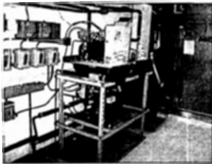
Water cooled Condensing units.
